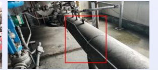
Fiber optic monitoring of pipeline vibration (sound)
