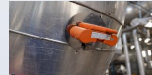
pipeline corrosion(52 positions)
